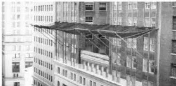
Nets must be installed in a manner that should an individual fall, they will not strike any object below the net (picture courtesy of DBI/Sala).
